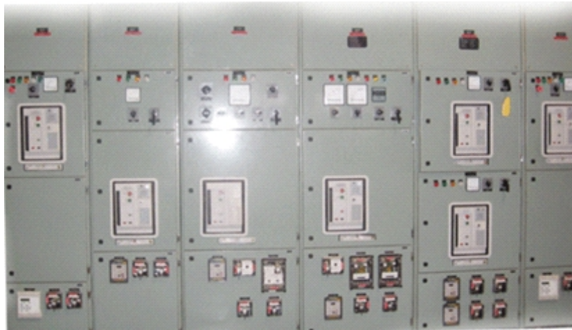
Fig 1.4.2: Power Control Centre
