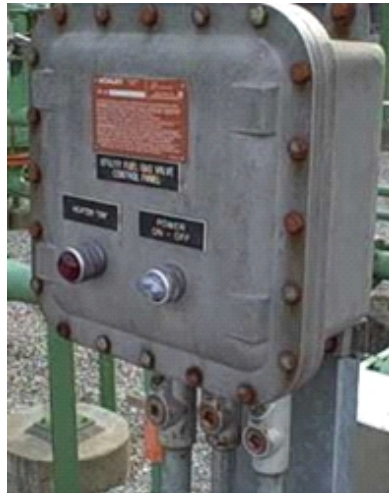
Fig 2.3.2.4: explosion proof enclosures
