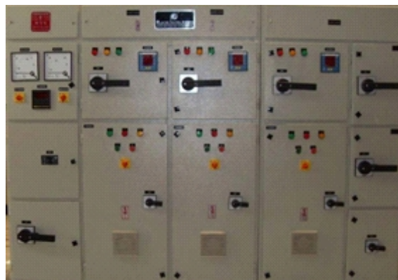
Fig 2.3.2.8: motor control centre
